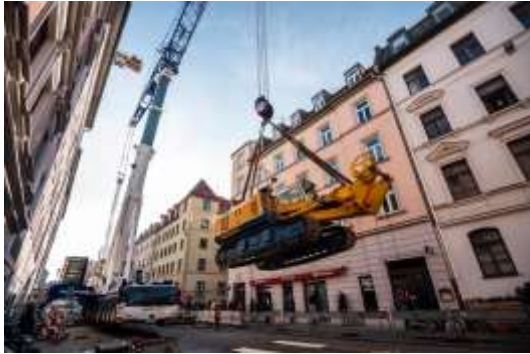
(1) The BG 20 H had to be lifted into the backyard by a truck-mounted crane.
