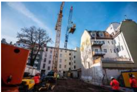
(3) A total of 348 piles with lengths between 8 and 13 m will be installed as a bored pile wall for the retaining structure using a BG 20 H.
